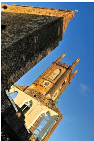
The remains of the severely hurricane-damaged Scottish Church, located in the island's capital city of St. George's.
